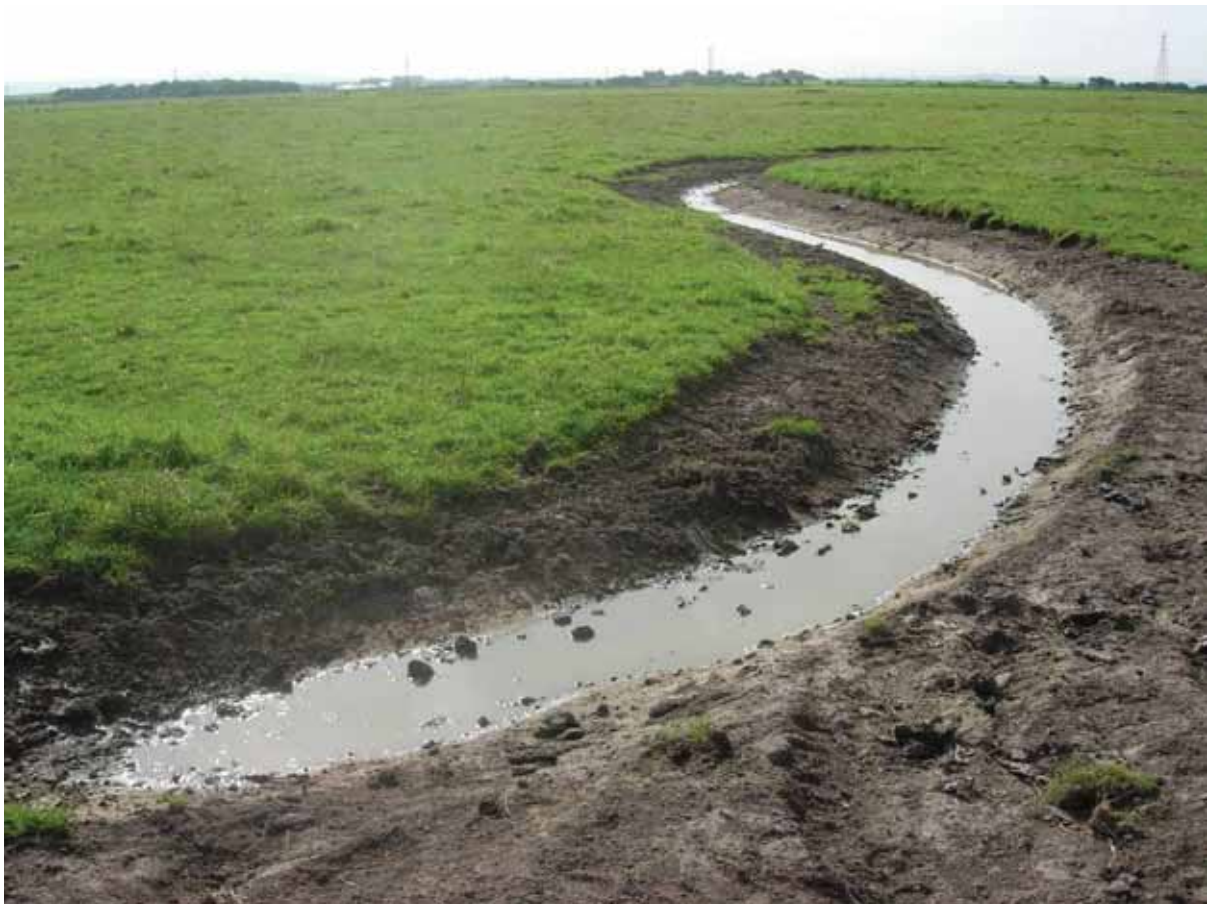
Newly created channel following rain a few weeks after the work © Andrew Gouldstone (RSPB)
