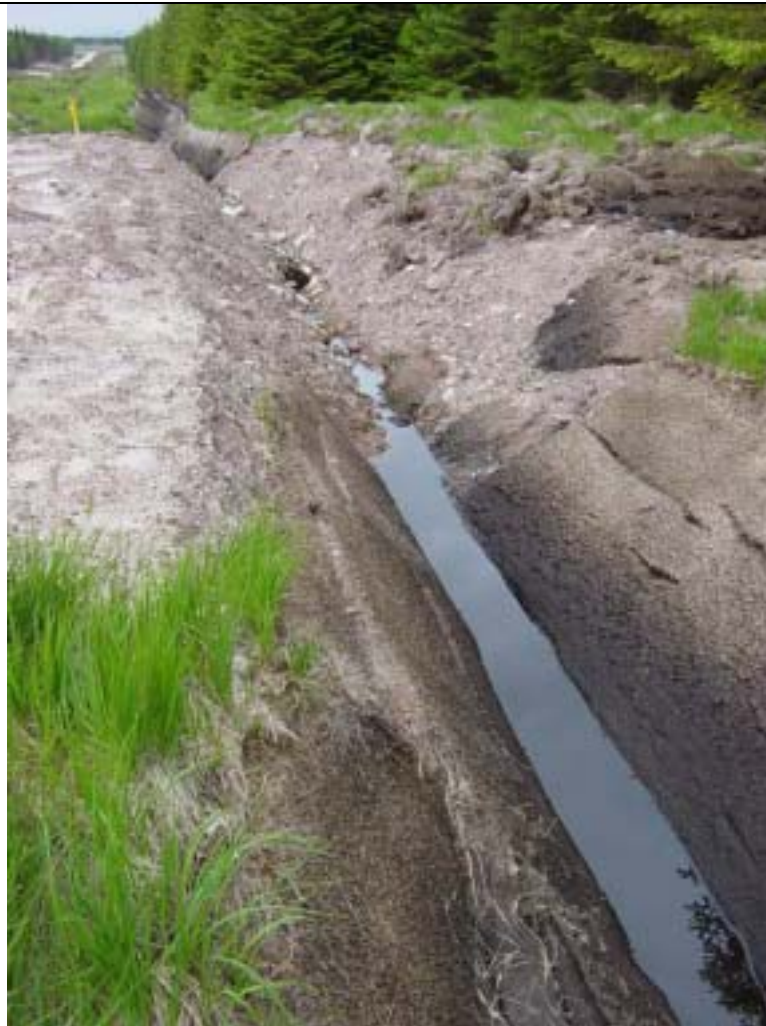
Figure 14. Drain installed after construction of the floating road visible on the left of the photograph. The road was constructed as part of a wind farm development at Derrybrien, Co. Galway, where the original proposal was for all roads to be undrained and floating on peat.
