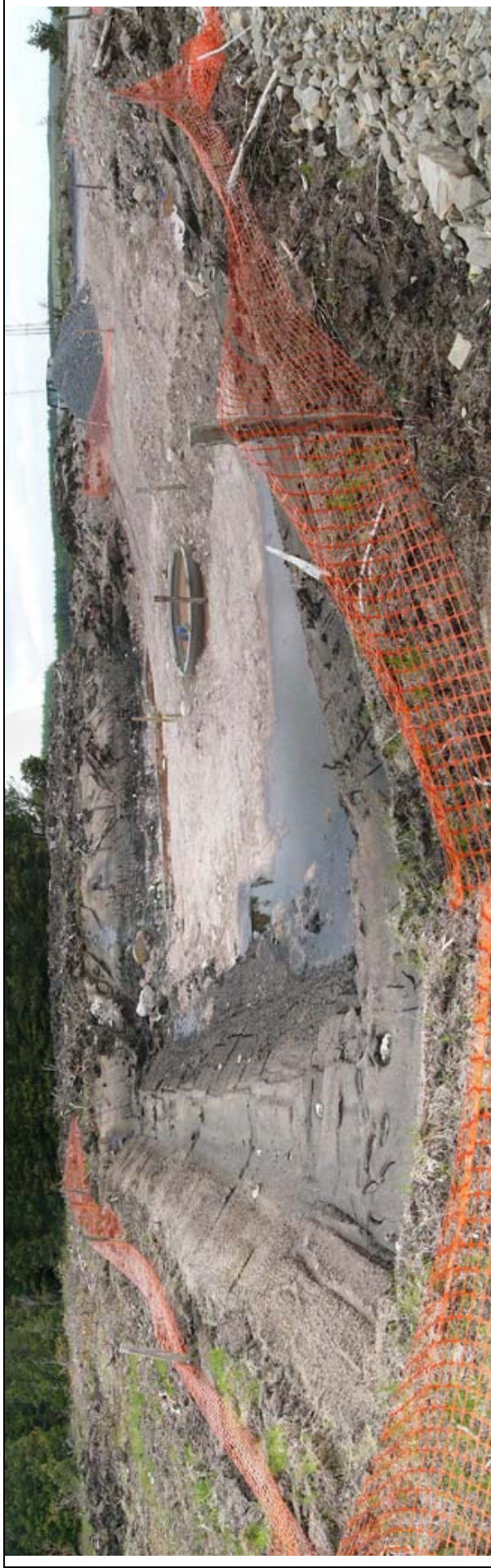
Figure 7. Panorama of turbine-base excavation at Derrybrien, Co. Galway, showing the extent of the excavation within the general blanket bog expanse. The turbine base, visible as the light green circle in the centre of the excavation bed, is approximately 4 metres in diameter. The dimensions of the excavation can thus be seen to be approximately 50 metres x 50 metres. The concrete base into which the base-can is set, is now buried beneath hardcore backfill, but is 15 metres x 15 metres. The size of base proposed for Lewis is significantly larger, at 22 metres x 22 metres.
