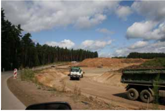
Białystok-Katrynka section of road no. 8 - under upgrading. Picture taken inside the Natura 2000 site, showing construction of the "Sochonie" road junction.
