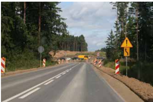
Białystok-Katrynka section of road no. 8 - under upgrading. Picture taken inside the Natura 2000 site, showing the "Sochonie" road junction.
