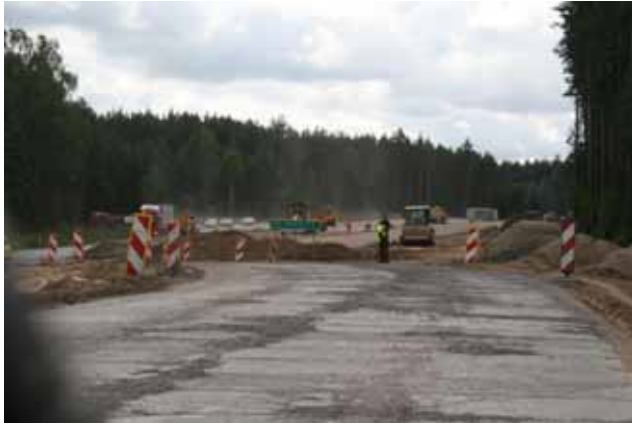
Białystok-Katrynka section of road no. 8 - under upgrading. Picture taken inside the Natura 2000 site.
