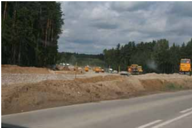
Białystok-Katrynka section of road no. 8 - under upgrading. Picture taken inside the Natura 2000 site.
