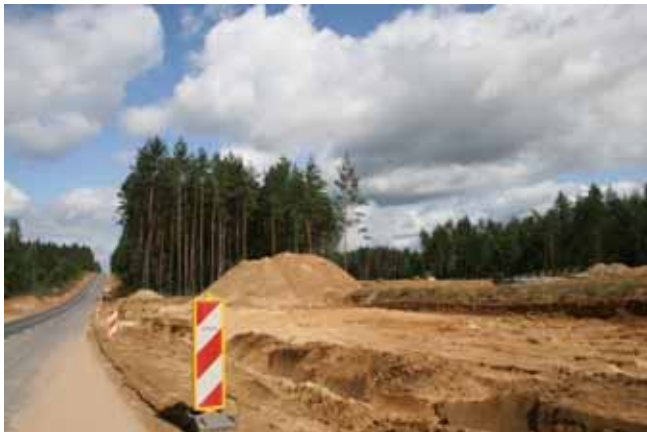
Białystok-Katrynka section of road no. 8 - under upgrading. Picture taken inside the Natura 2000 site.
