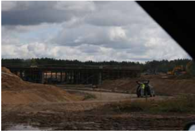
Białystok-Katrynka section of road no. 8 - under upgrading. Picture taken inside of the Natura 2000 site, showing construction of the "Sochonie" road junction construction and the planned connection with Wasilkow Bypass.
