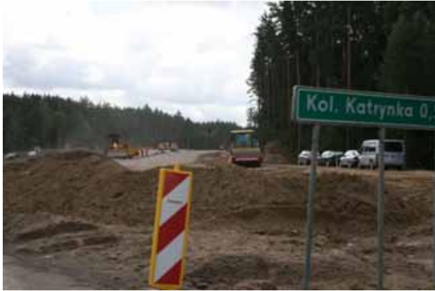
Białystok-Katrynka section of road no. 8 - under upgrading. Picture taken inside the Natura 2000 site.
