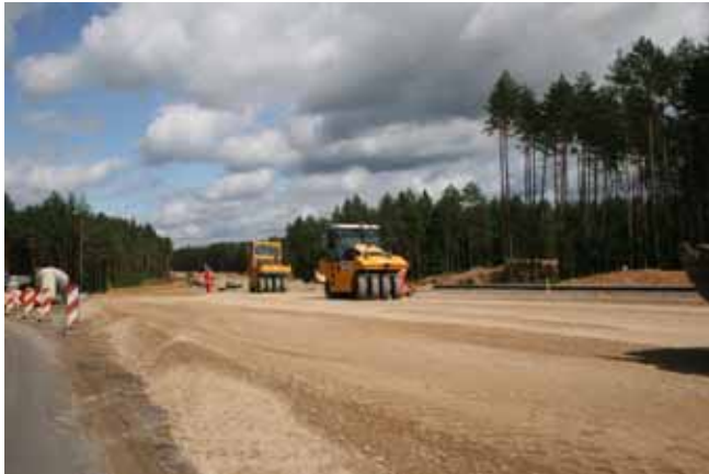
Białystok-Katrynka section of road no. 8 - under upgrading. Picture taken inside the Natura 2000 site.
