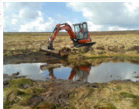
Machinery is used to shape pool edges to allow easier access for birds to feed.
